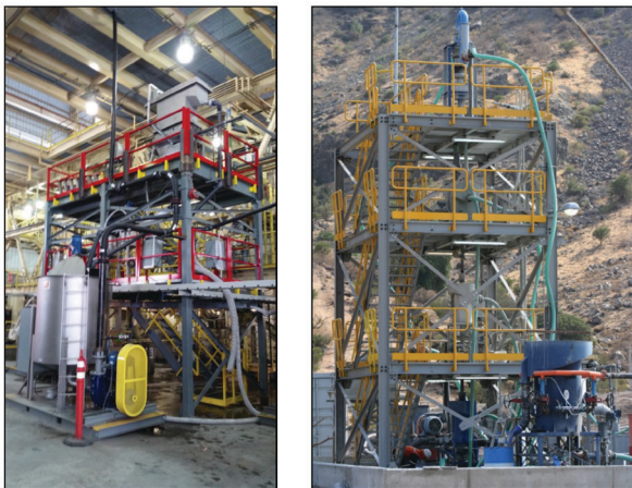
Figure 10 Installation photos for Eriez split-feed pilot plant.
